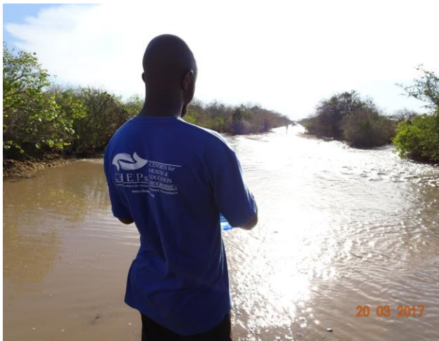
Flooded section of the road
