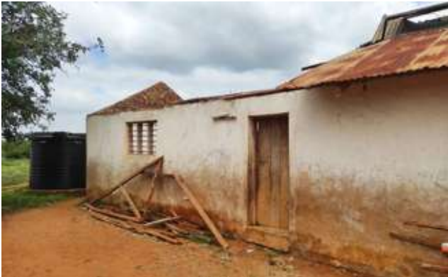
Classroom with roof destroyed
