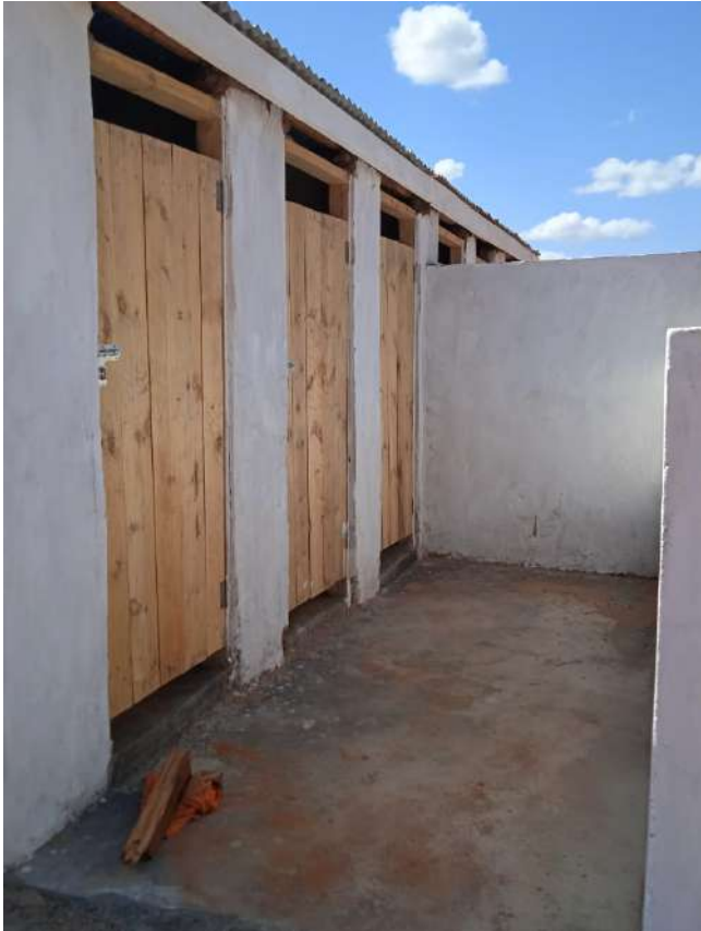
3 cubicles for boys and 3 for girls partitioned to ensure privacy
