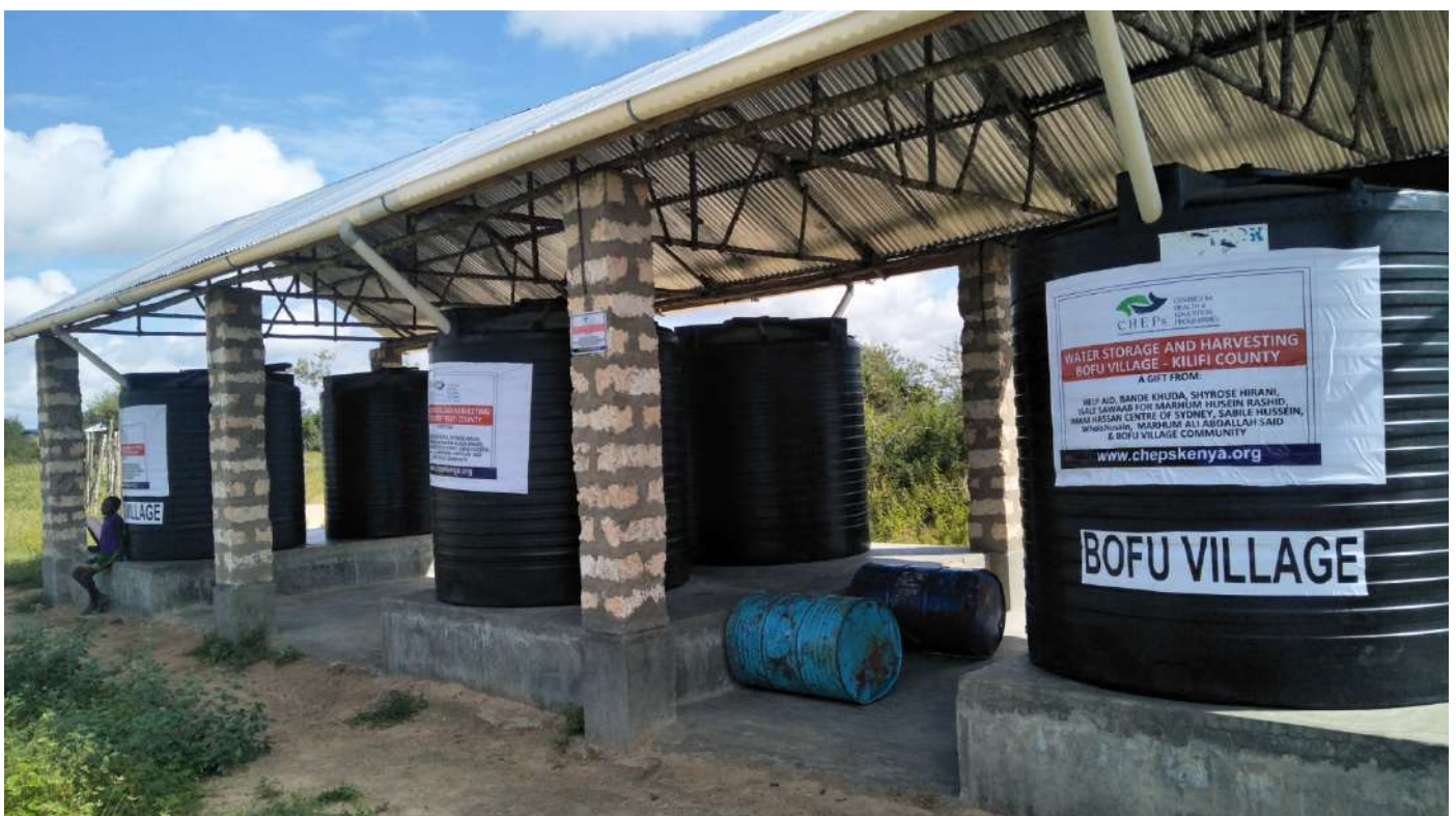
The rain water harvesting tanks constructed at Bofu village in 2018
